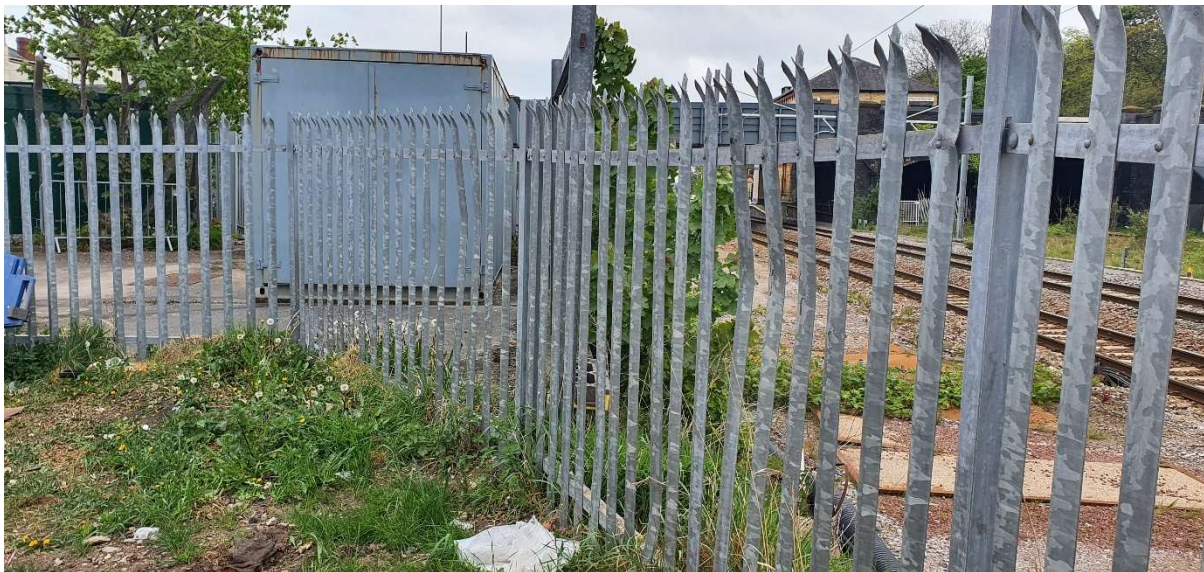
At the vehicle entry point – approximate drop of 400mm down to lineside
