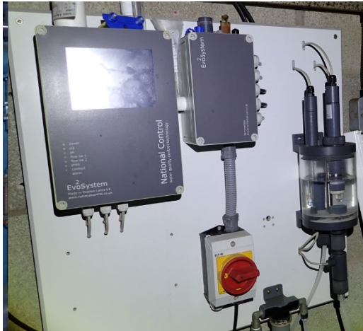
EVO 2 Controls System
