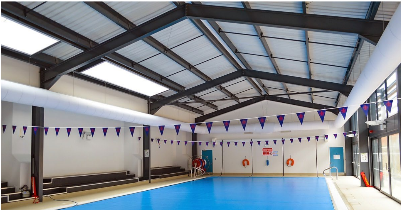
Typical Textile Ventilation Duct to Pool Hall
