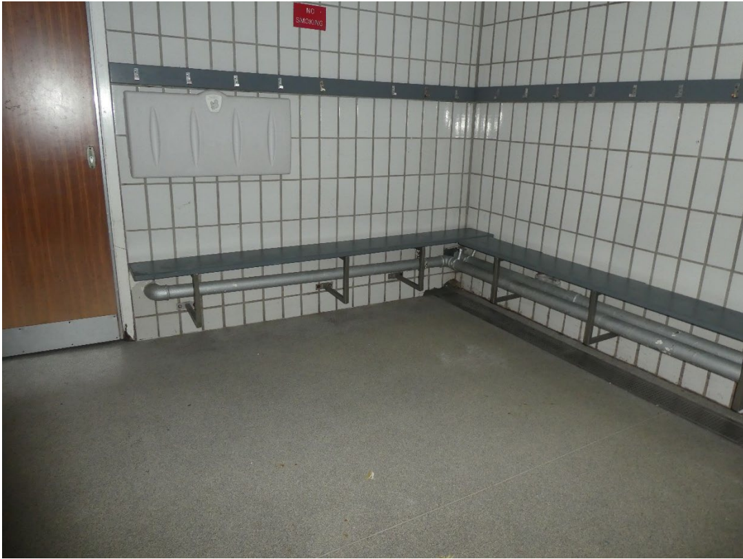
Typical Pipe Heating Coil Under Benches
