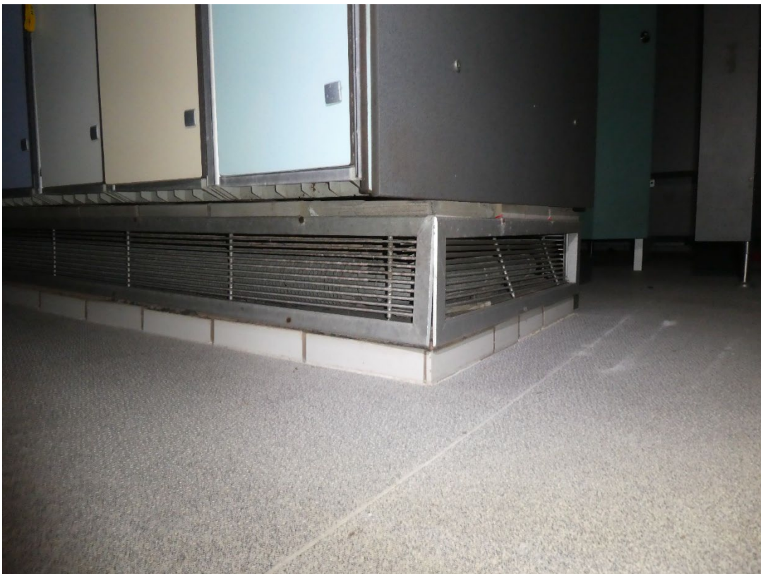
Typical Finned Tube Heaters to Lockers
