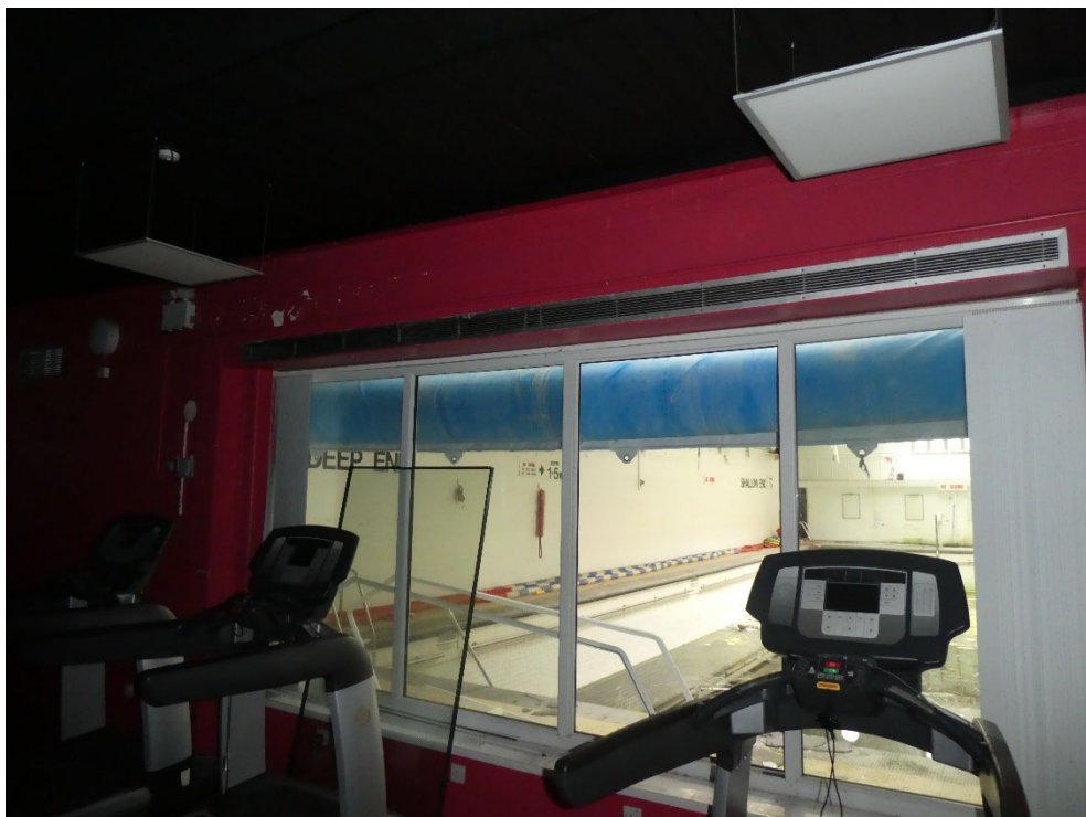
High Level Supply Air Grilles in the Gym
