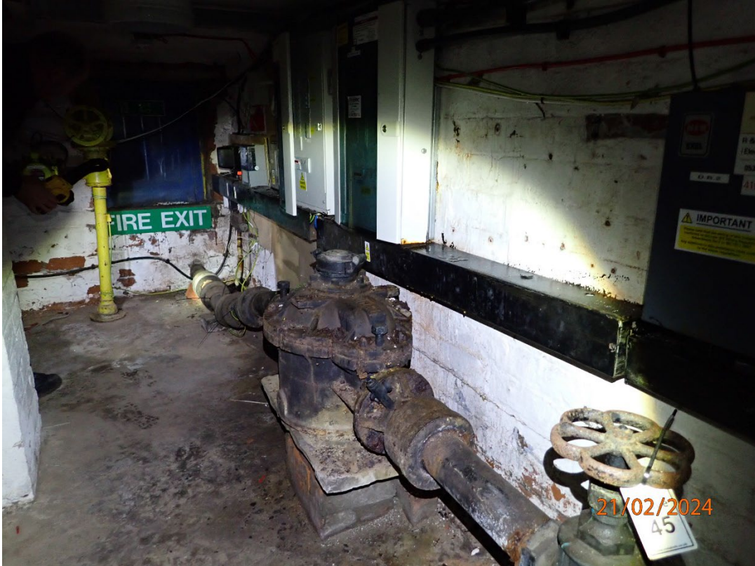
Utility Company's Mains Cold Water Meter Assembly
