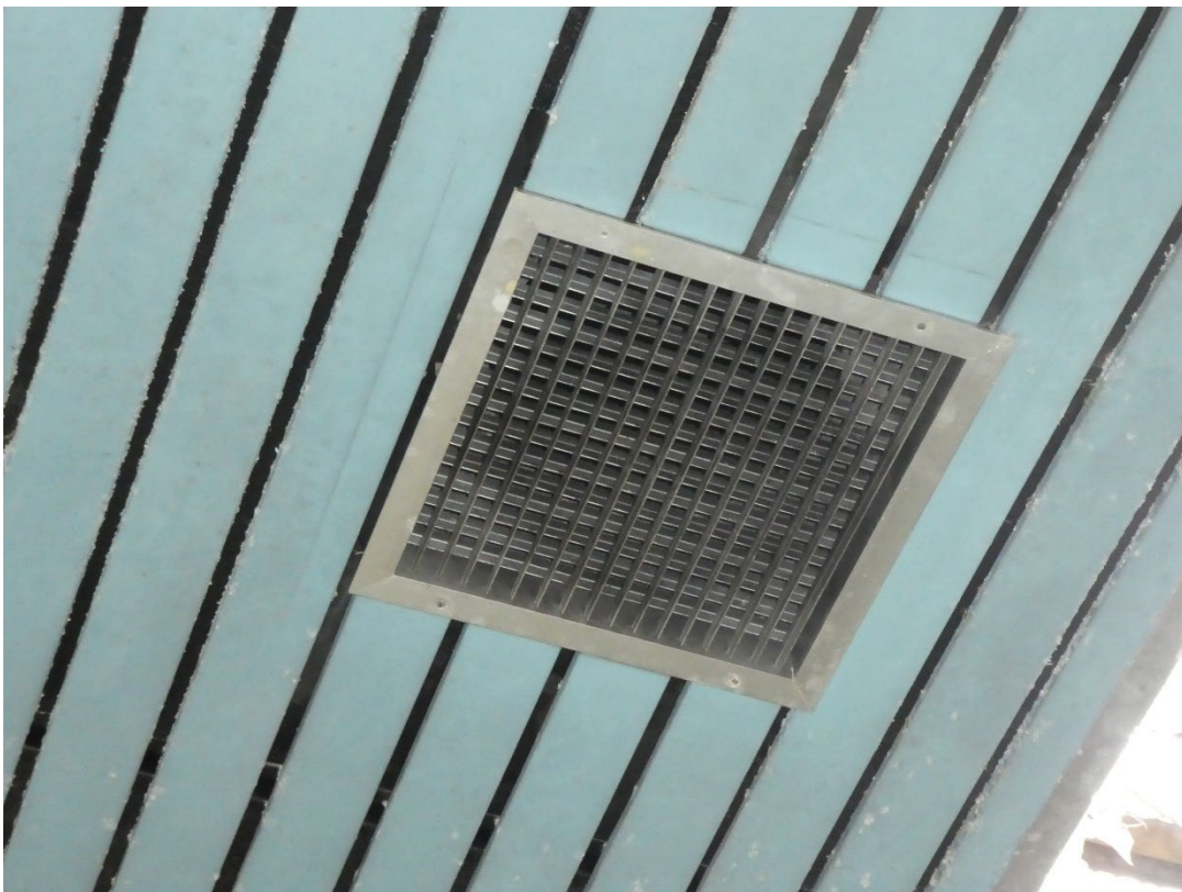
Pool Area Supply Grille
