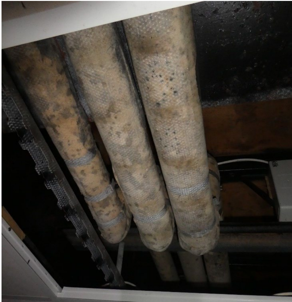
Typical Pipework Installation in Ceiling Void
