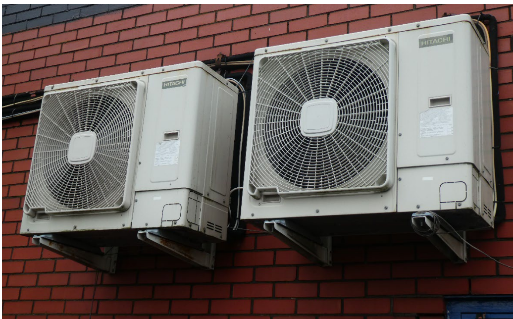
Gym AC Outdoor Units
