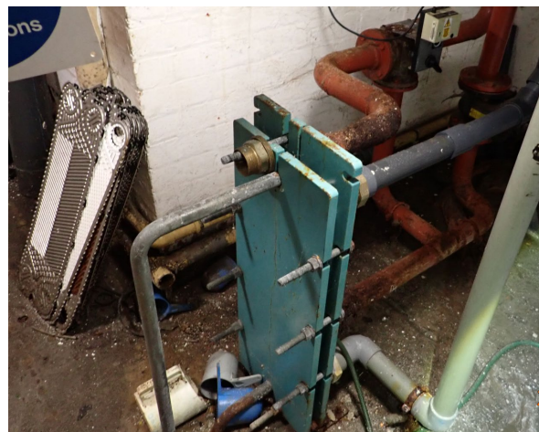
Pool Heat Exchanger
