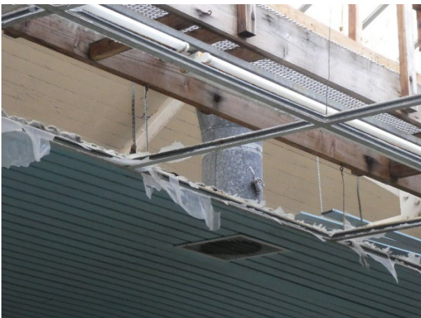
Swimming Pool Roof Void Lighting
