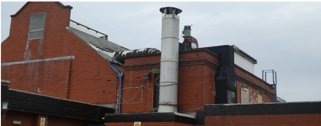
LTHW Boiler Plant Combustion Exhaust Flue
