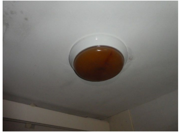
Disabled WC Lighting
