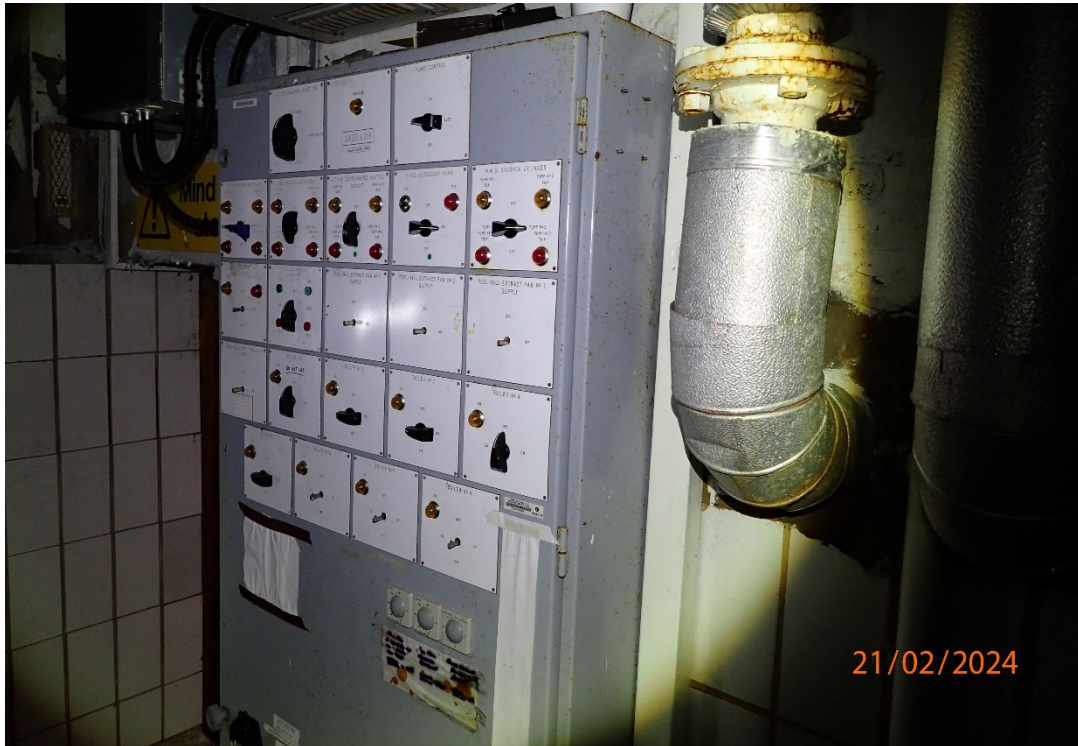
HVAC Control Panel
