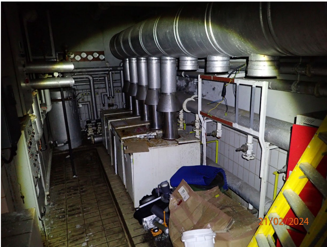
LTHW Boiler Plant
