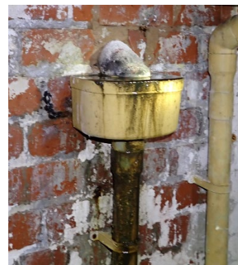
Existing Pool Skimmer Hoppers
