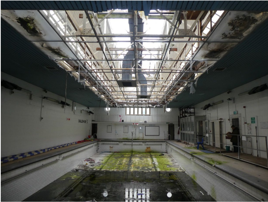
Pool Area Ductwork
