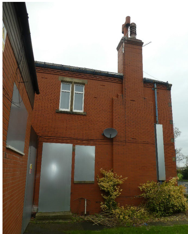
Incoming Natural Gas Service to Two-Storey "House" Area
