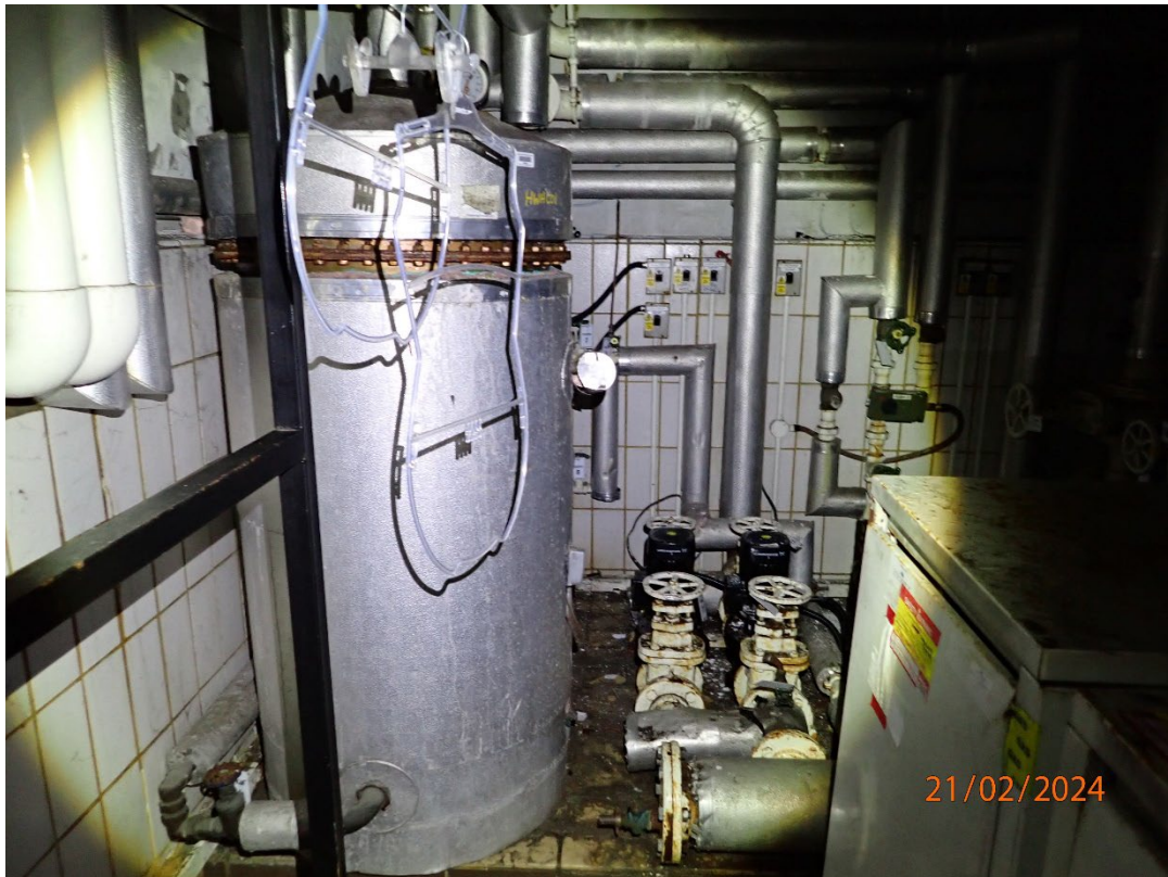
HWS Storage Calorifier
