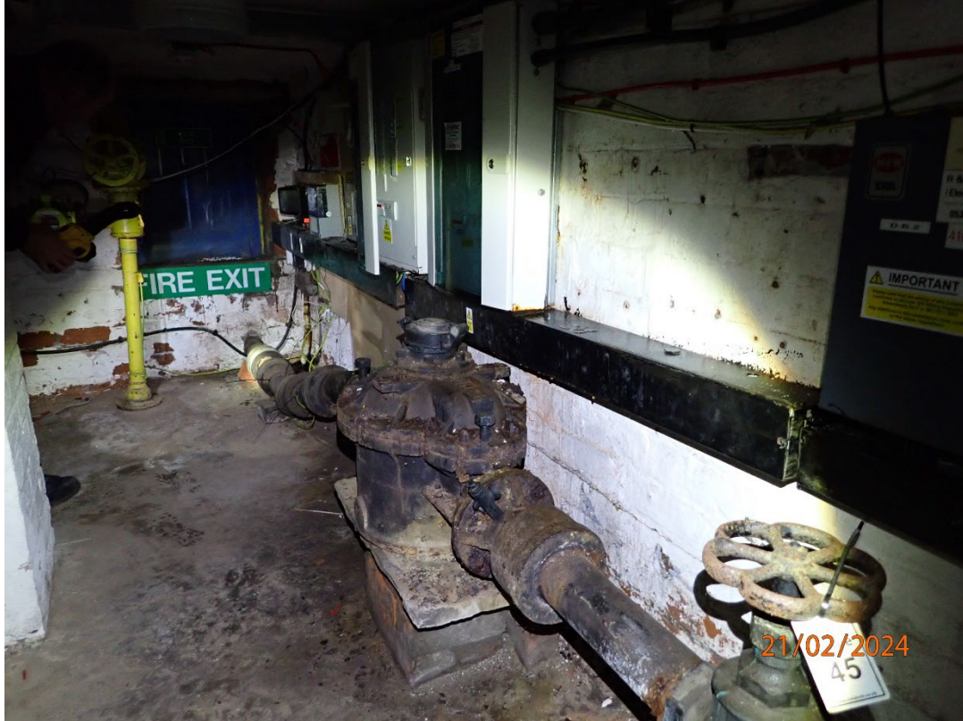
Utility Company's Mains Cold Water Meter Assembly
