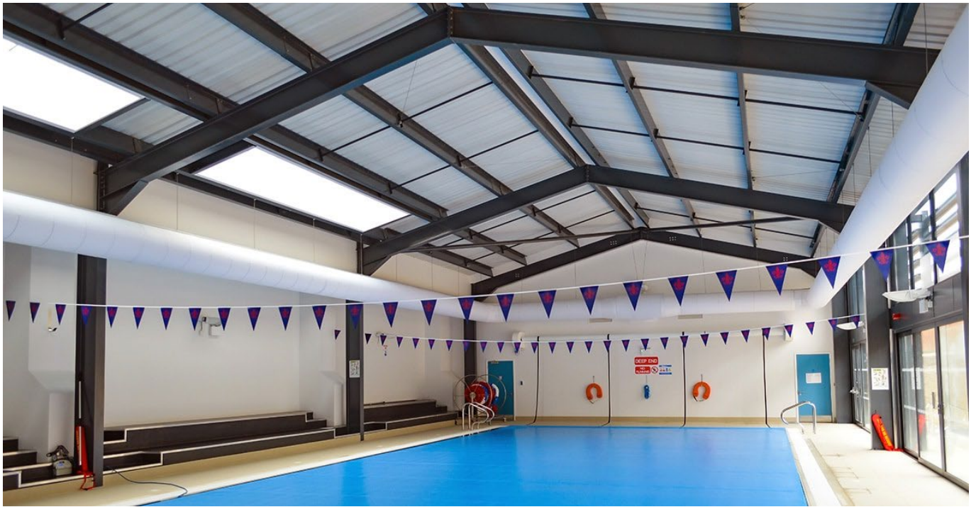
Typical Textile Ventilation Duct to Pool Hall
