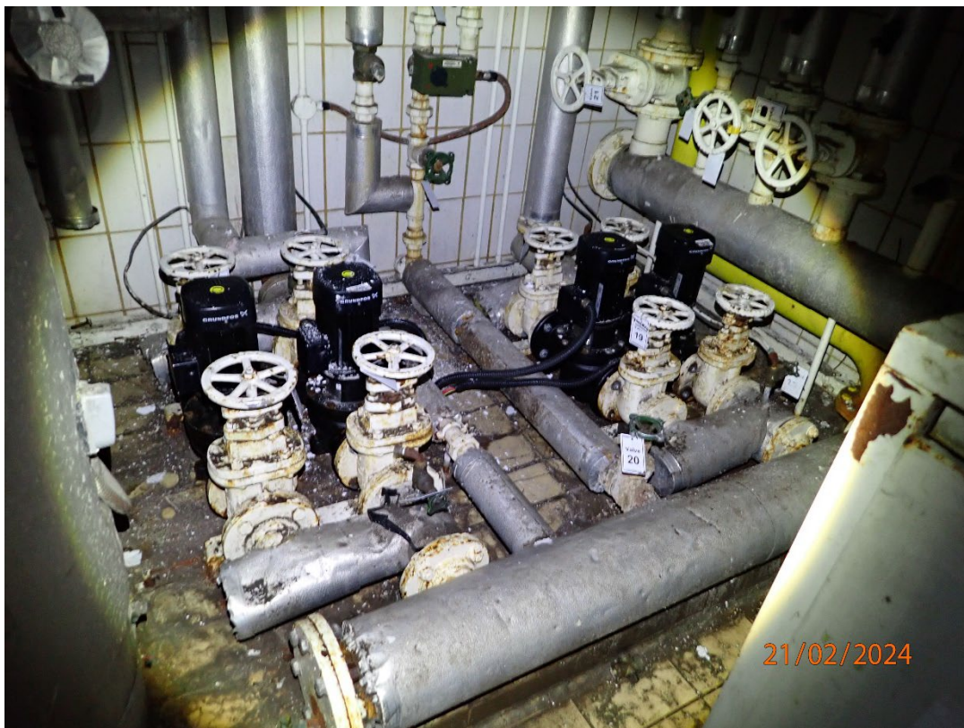
Typical Heating System Pumps
