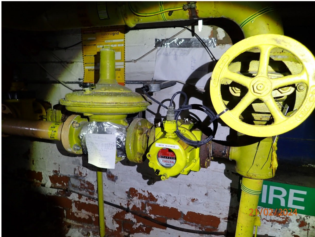
Utility Company’s Natural Gas Service Governor & Meter Assembly
