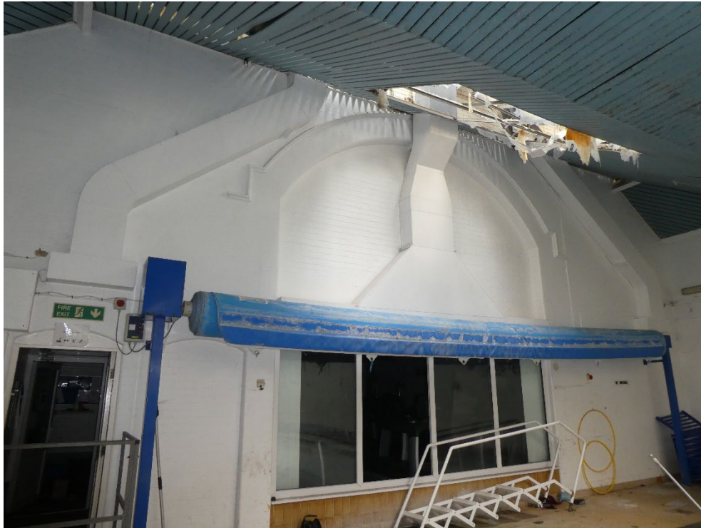
Ductwork Serving the Gym (Routed on the Wall)
