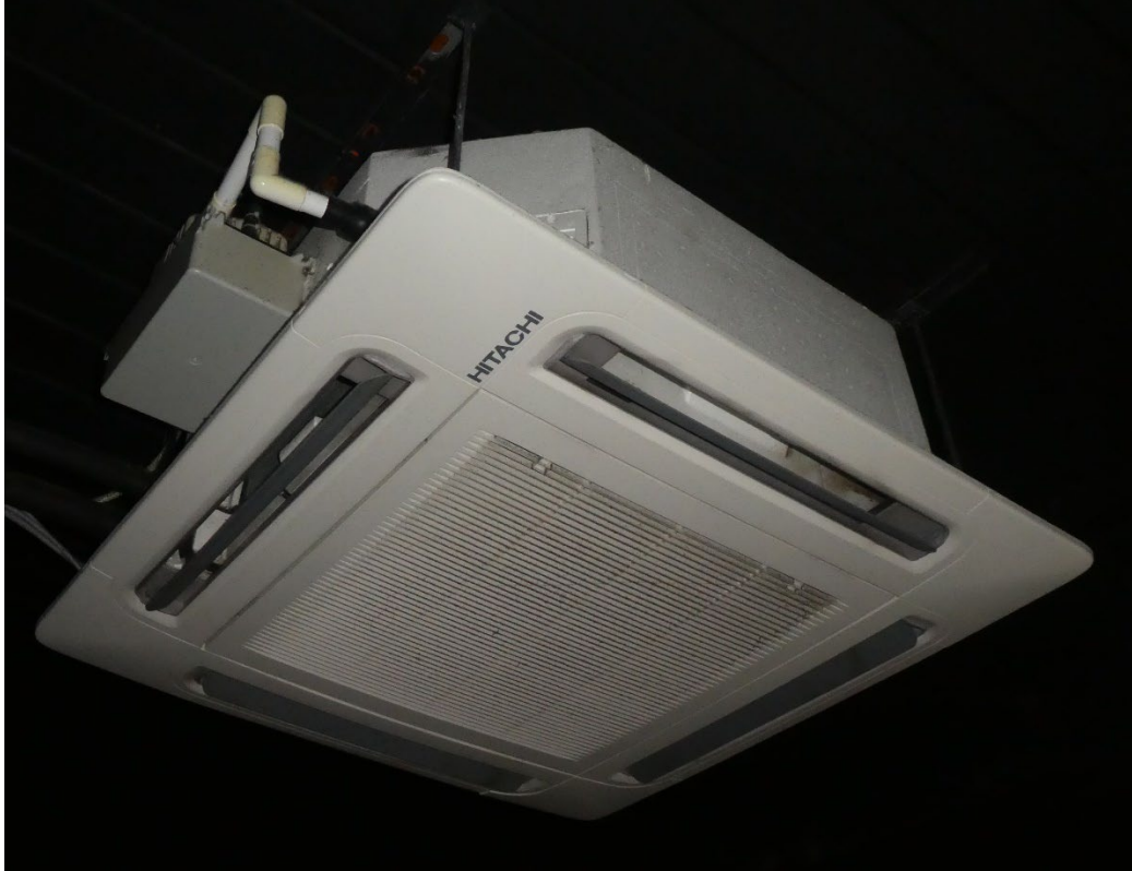
Gym AC Indoor Unit
