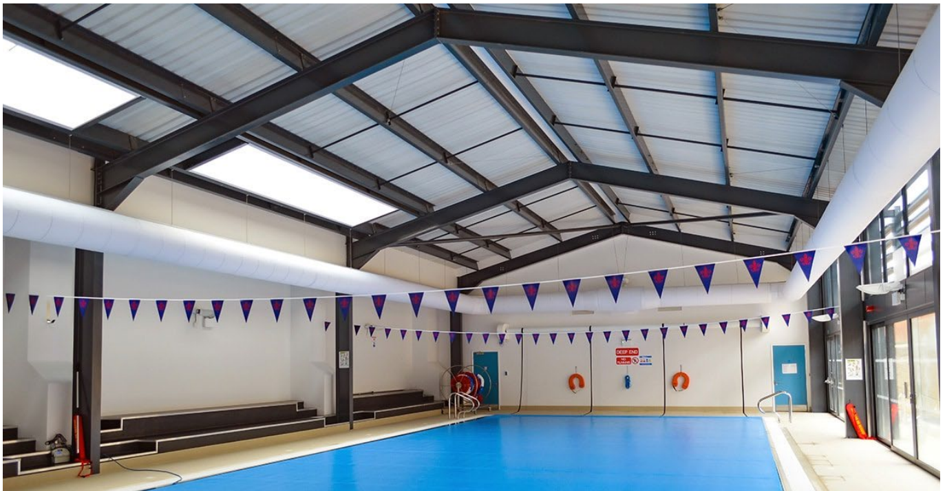
Typical Textile Ventilation Duct to Pool Hall
