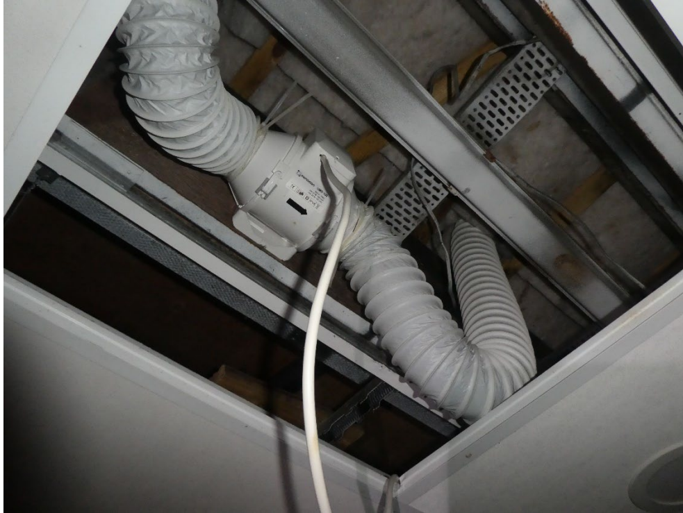
Local Ducted Extract Fan (Female Changing Area)
