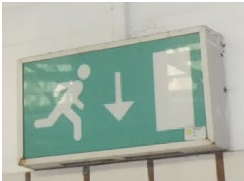
Typical Emergency Exit Luminaire
