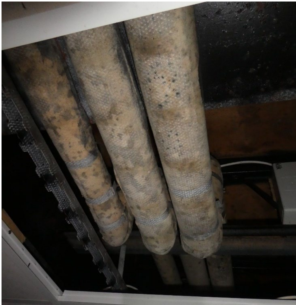
Typical Pipework Installation in Ceiling Void
