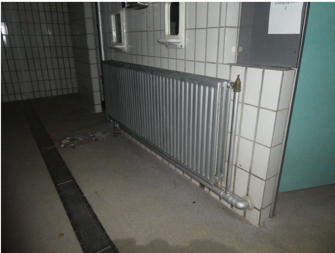
Typical Pressed Steel Panel Radiator (Painted Silver)
