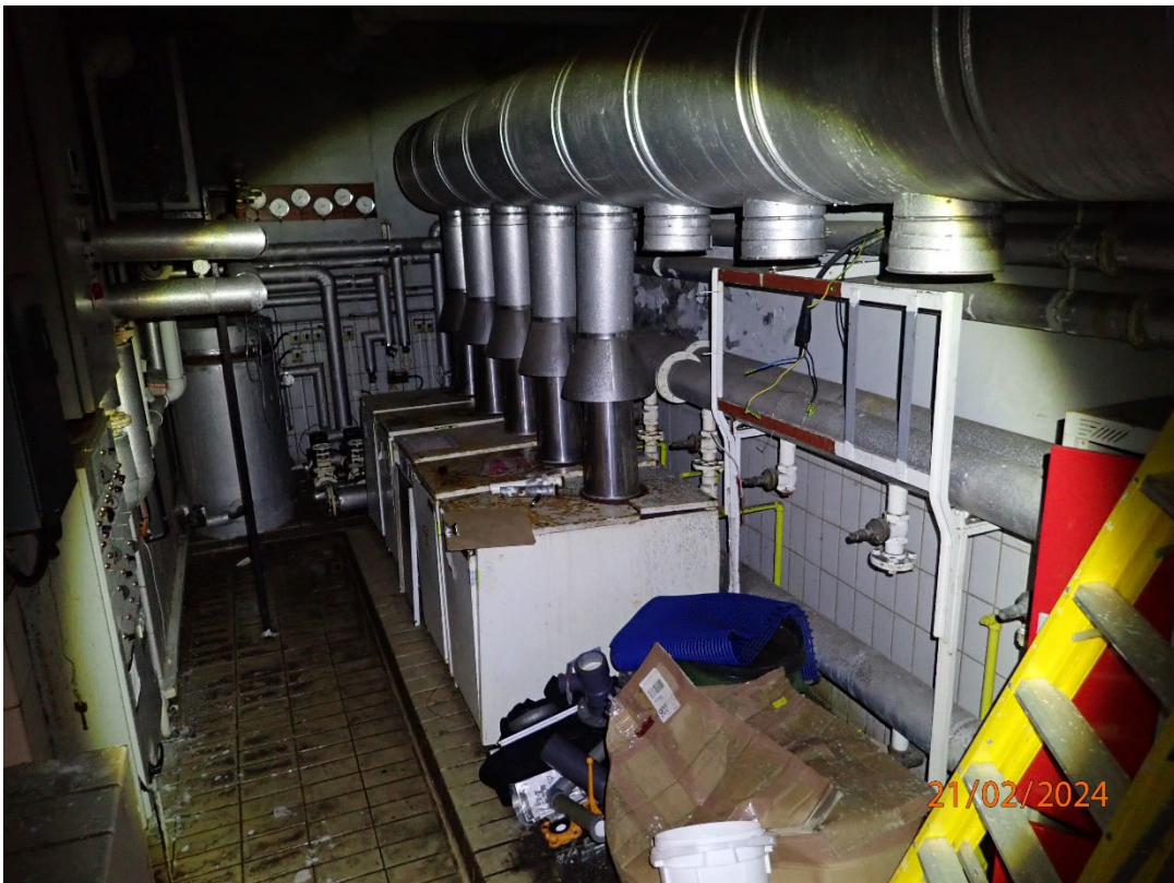
LTHW Boiler Plant
