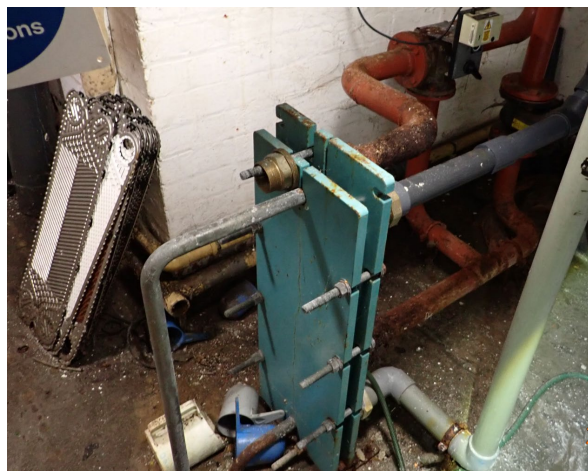
Pool Heat Exchanger
