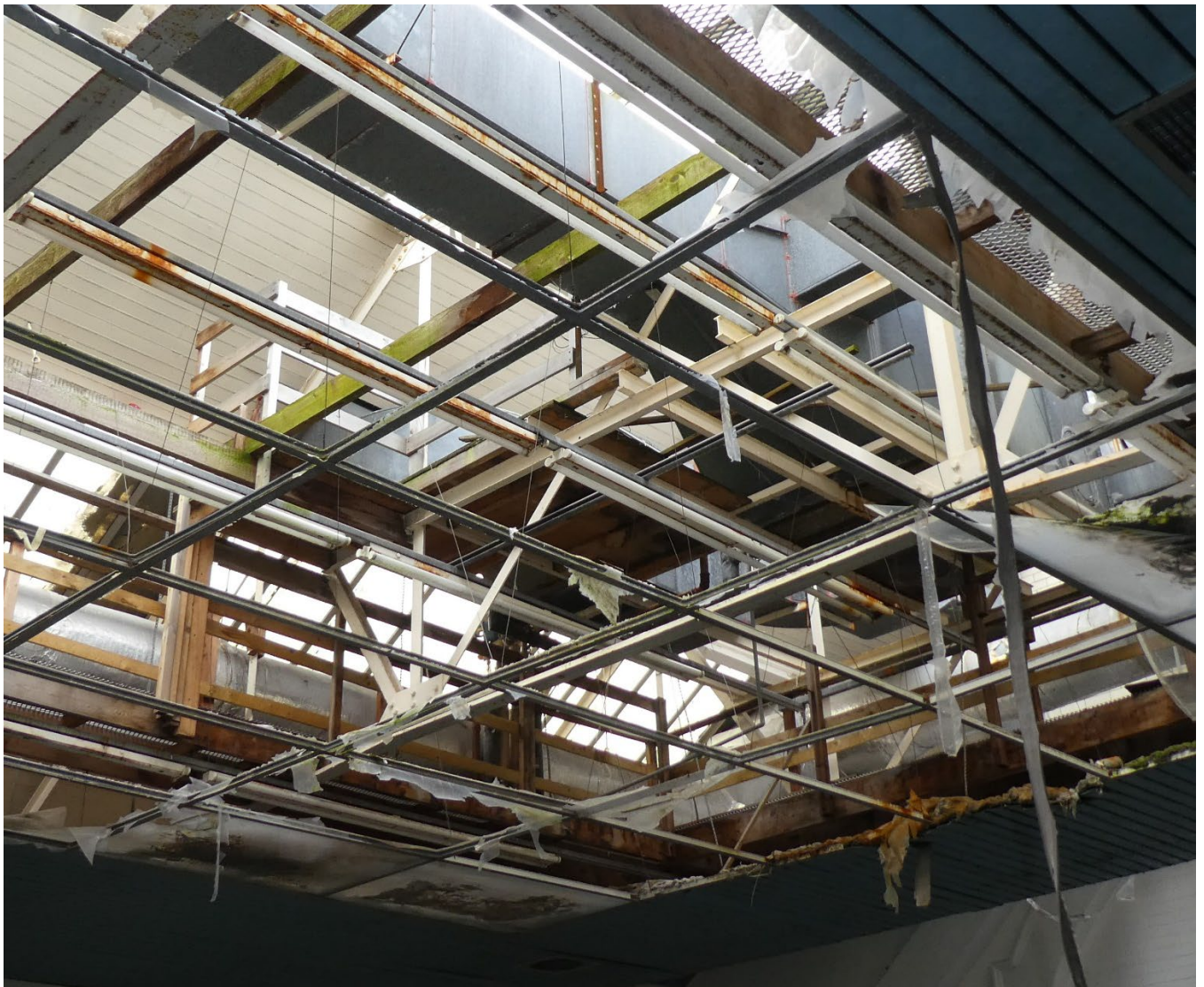
Pool Area AHU
