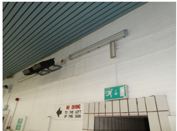
Swimming Pool Lighting
