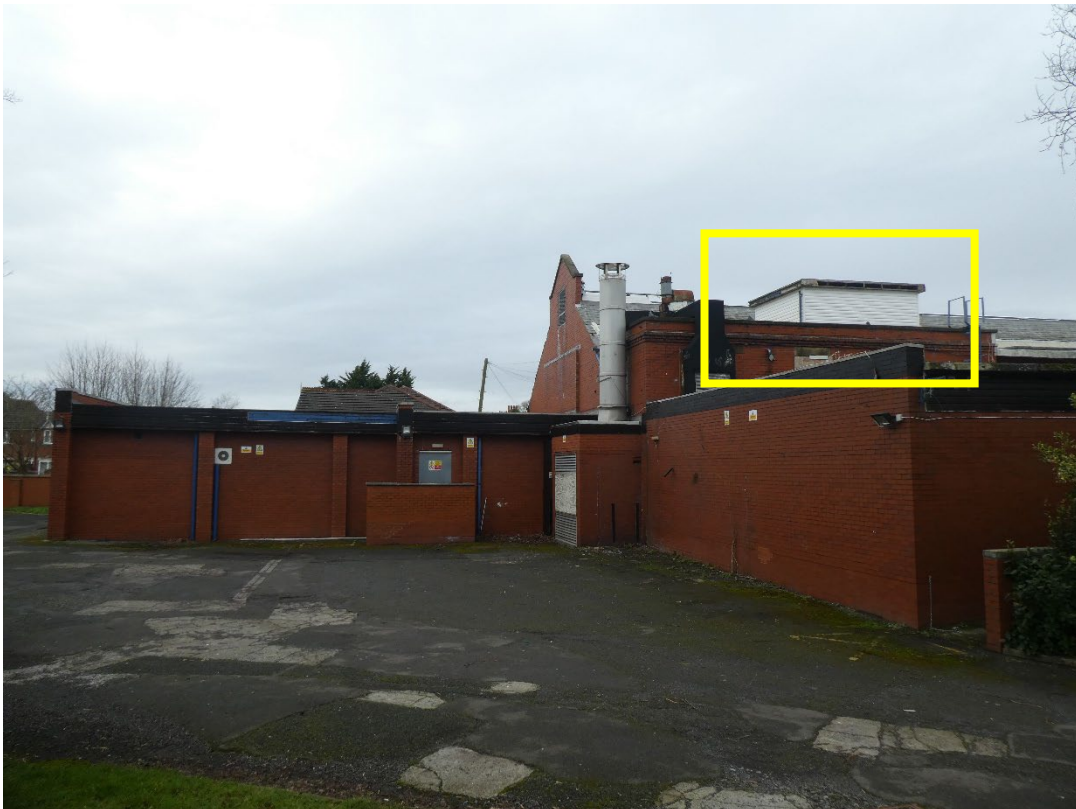
Rooftop Enclosure for Potable Cold Water Storage Cistern(s) Enclosure Clad in White Panelling (Highlighted in Yellow Box)
