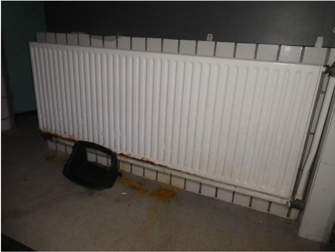
Typical Pressed Steel Panel Radiator (Rust along Bottom Edge)
