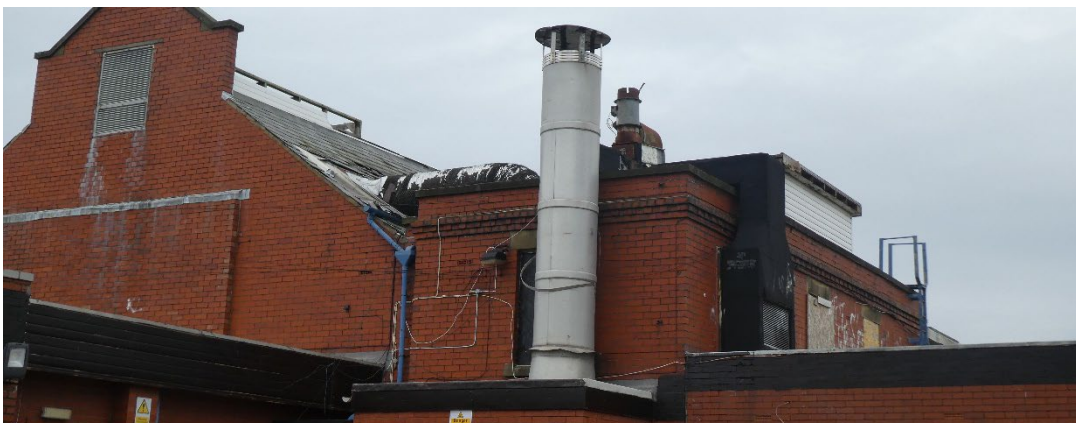
LTHW Boiler Plant Combustion Exhaust Flue
