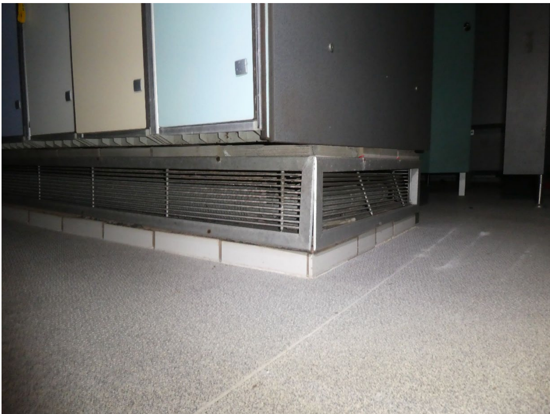
Typical Finned Tube Heaters to Lockers
