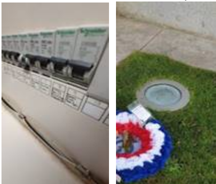
Distribution equipment and water ingress to luminaries
