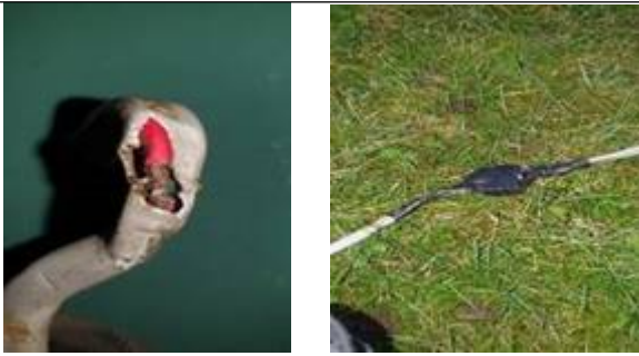
Damage to cable inside the column including evidence of previous repairs
